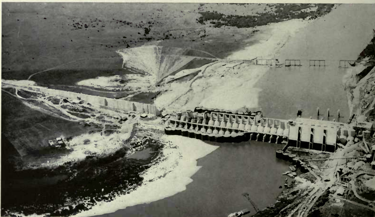
Construction of hydroelectric plant in Uruguay for which U. S. Steel supplied numerous steel products.
